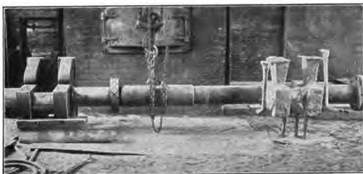
FIG 96.—The completed weld made by the use of thermit as in Fig. 95.
